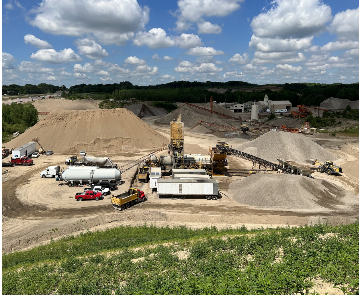
Temporary Portable Concrete Plant
